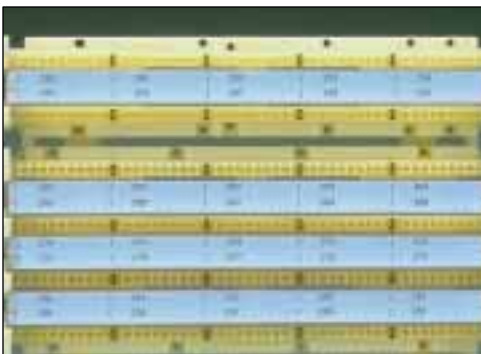
Network Systems Labeling
