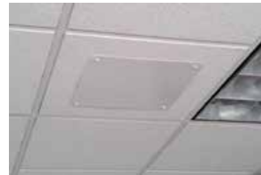
Installed Condition: PSIBVHF and PSIBVU78
