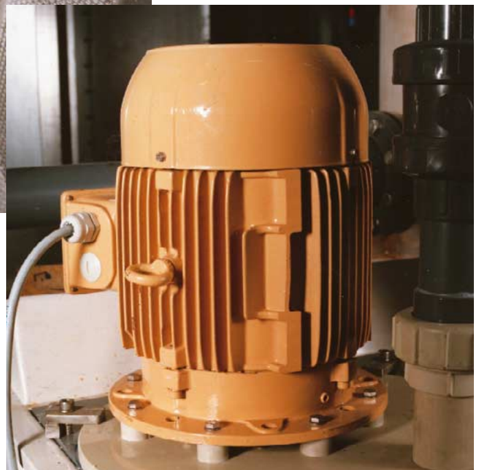
Monitoring a pump in a sewage treatment plant
